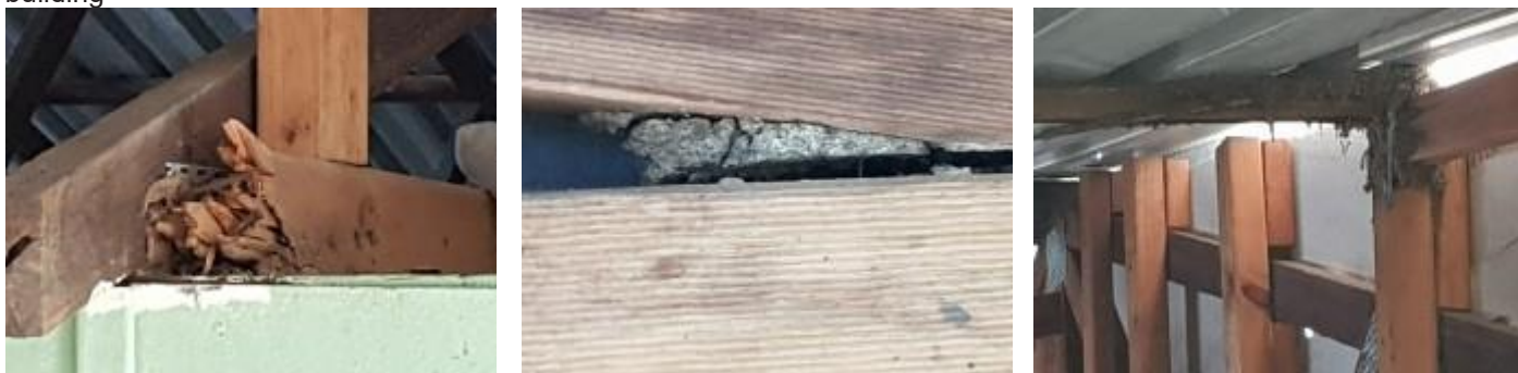
Extensive structural damage 2 old shed building
